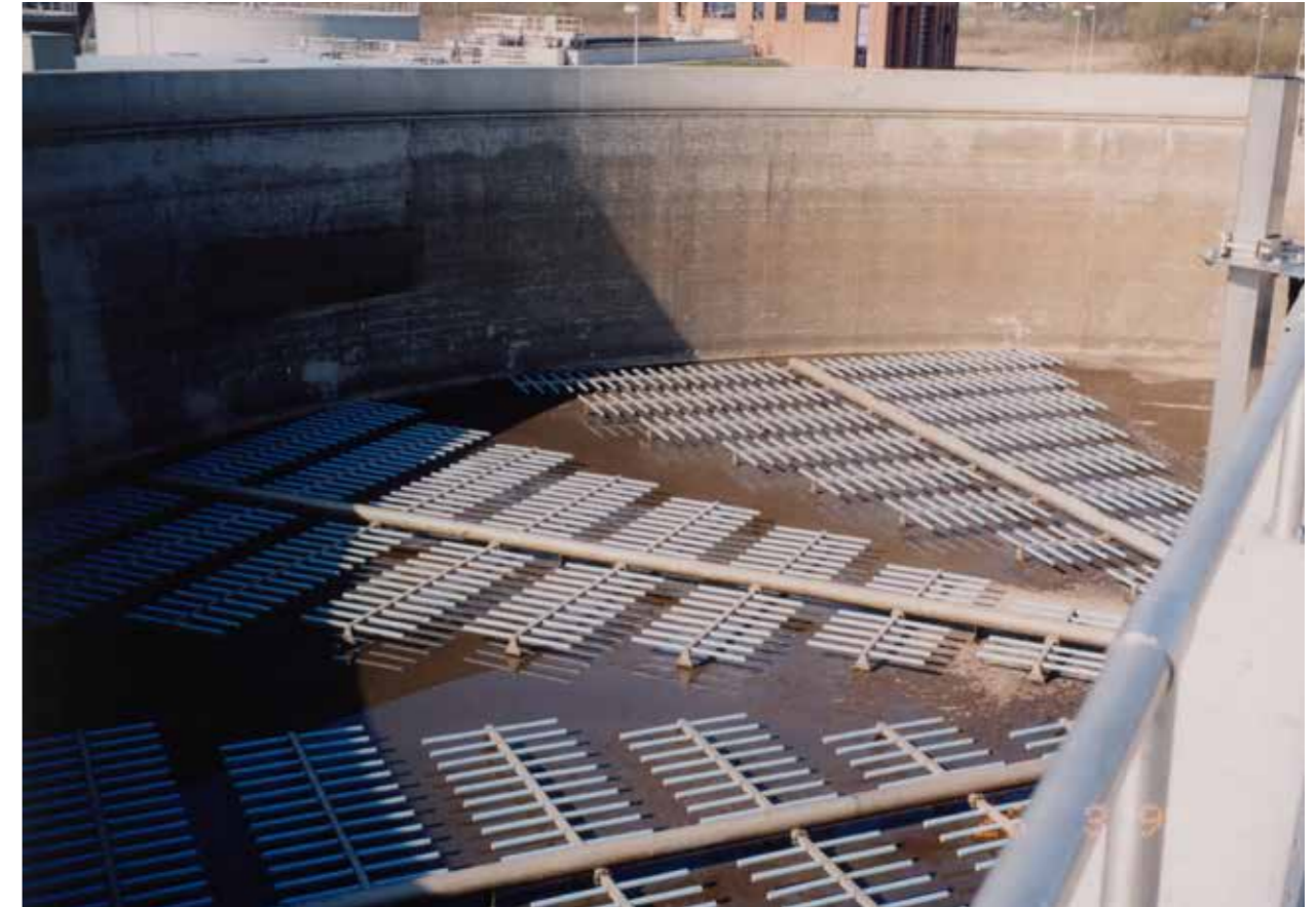
BUTTING pipes for a better quality of life, here in a sewage treatment plant
